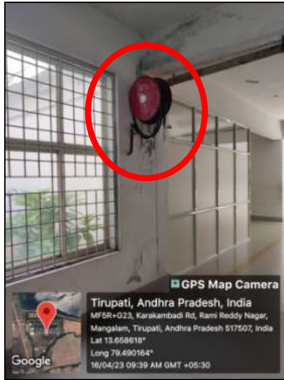
Firefighting equipment in Ground Floor
