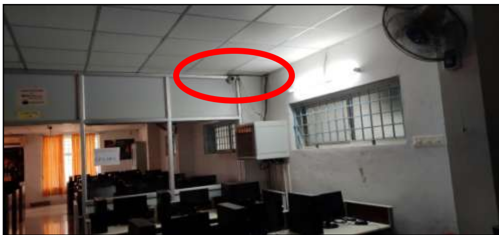
CC Cameras installed in Laboratory
