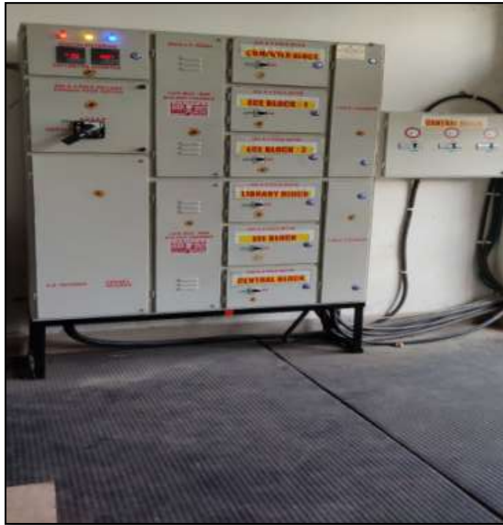
MCB' installed for Electric Safety and Insulated Mat Provided
