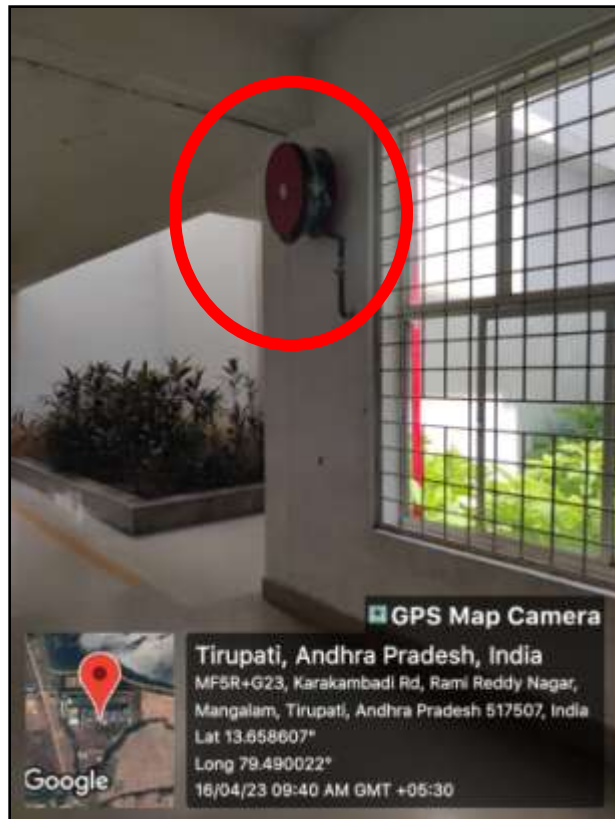
Firefighting equipment in First Floor
