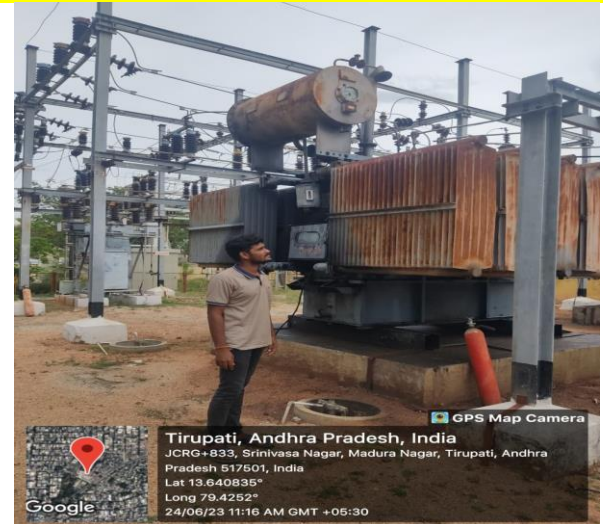
33/11 kV substation at Tirupati
