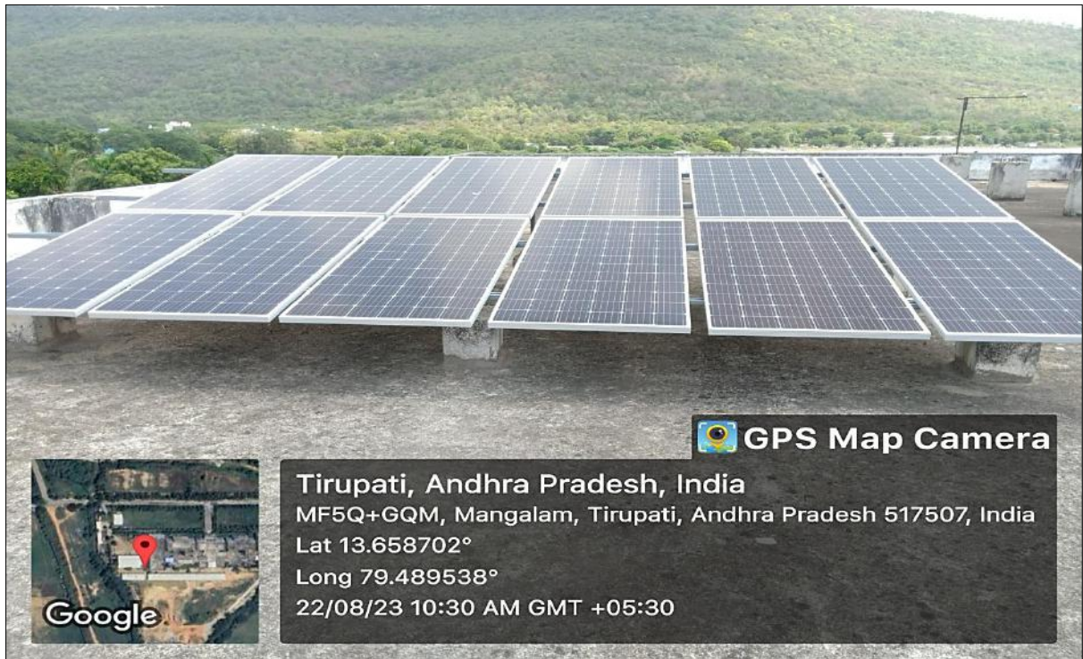
Solar Plant at Roof Top
