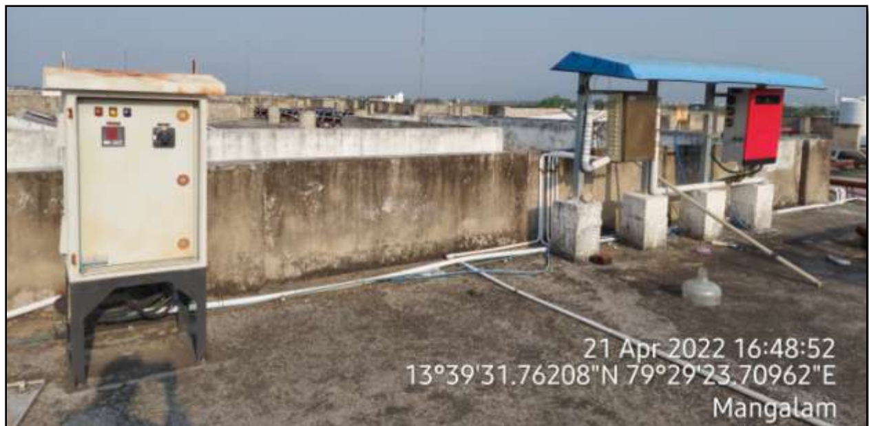
Solar Grid Connection
