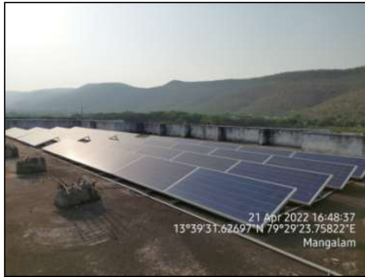
Solar Rooftops in the College Building
