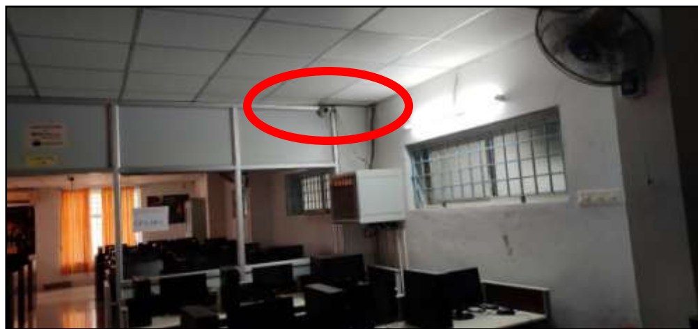
CC Cameras installed in Laboratory
