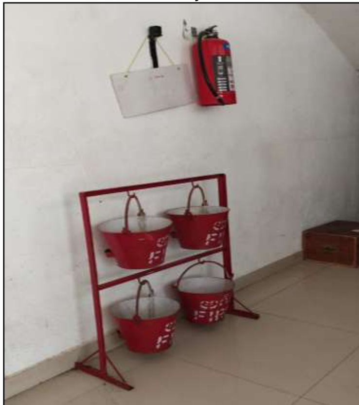
Fire Extinguisher and Sand Buckets for Fire Safety
