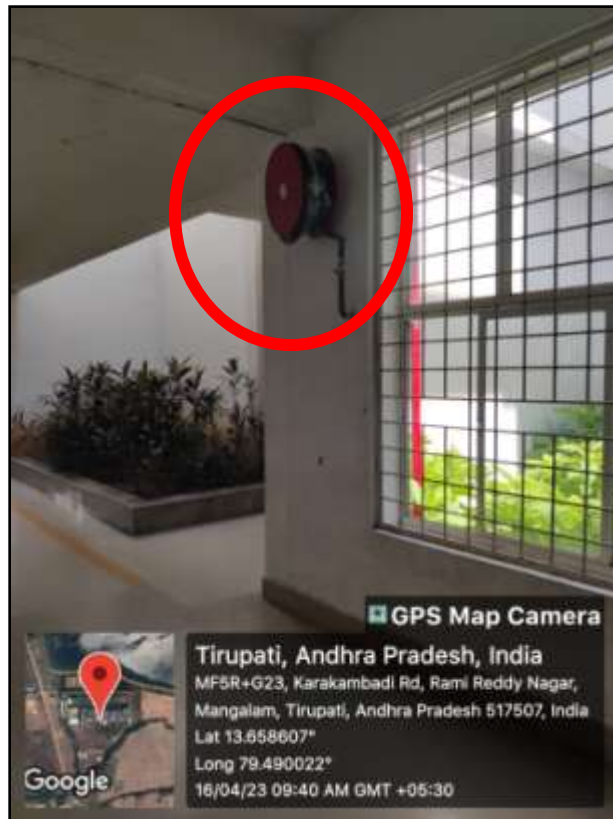
Firefighting equipment in First Floor
