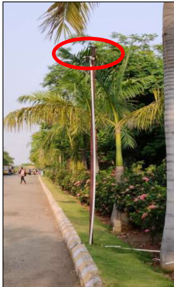
CC Cameras installed at the Main gate
